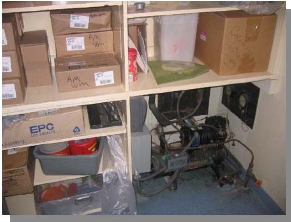
Water Cooled Compressor for Walk-in Refrigerator with an Open Continuously Wet Drain in the Dry Food Storage Area - Insect and Rodent Risk at AM Winn Elementary and Multiple School Sites
