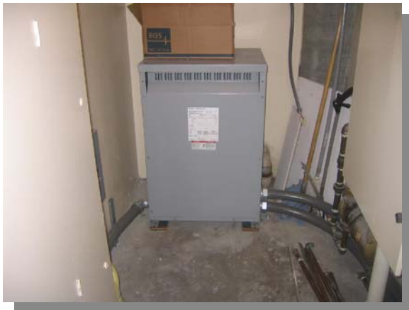
New Transformer Providing Power to the West Wing
