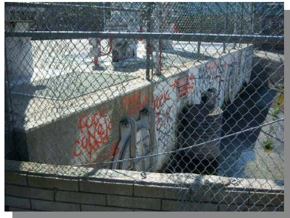
Damaged Fencing near Pump Station at CB Wire ES
